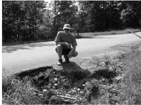
Michael Dixon observes roadside erosion
